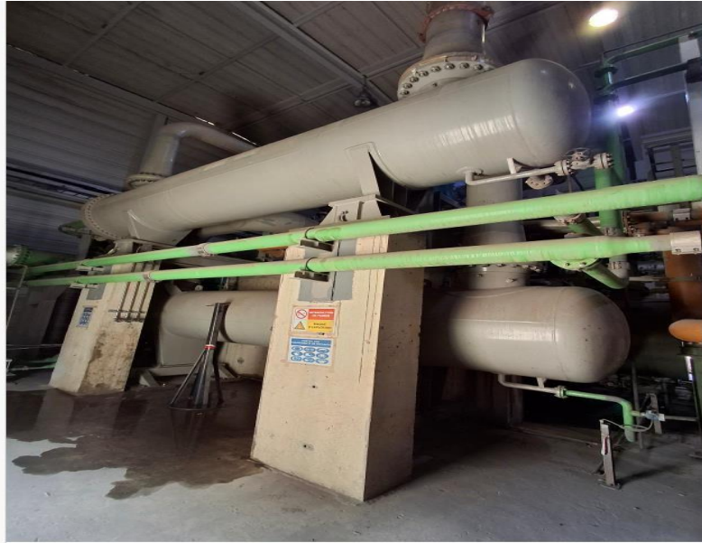
Appendix D.3: Real picture of the Main AIR Compressor
