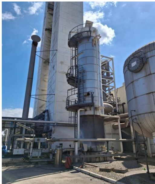
Appendix D.8: Real picture of the evaporation cooler
