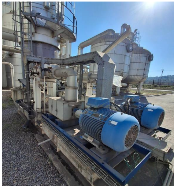
Appendix D.12: Chilled water pumps
