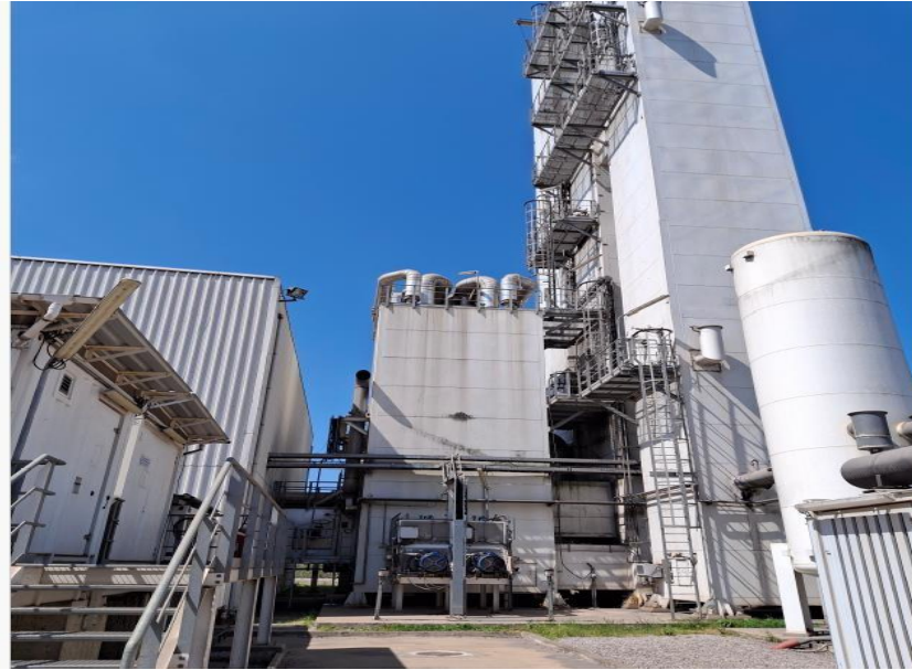
Appendix D.5: Real Picture of the main Heat exchanger
