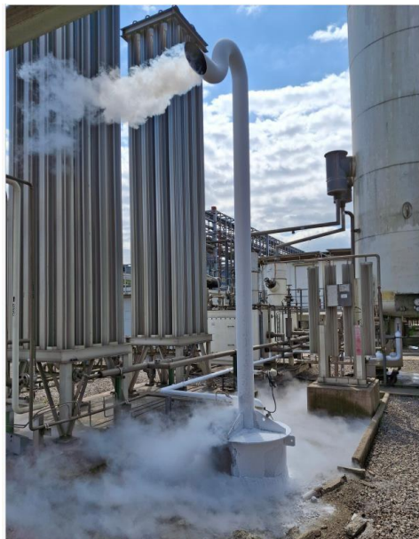
Appendix D.6: Real Picture impure Nitrogen Drain
