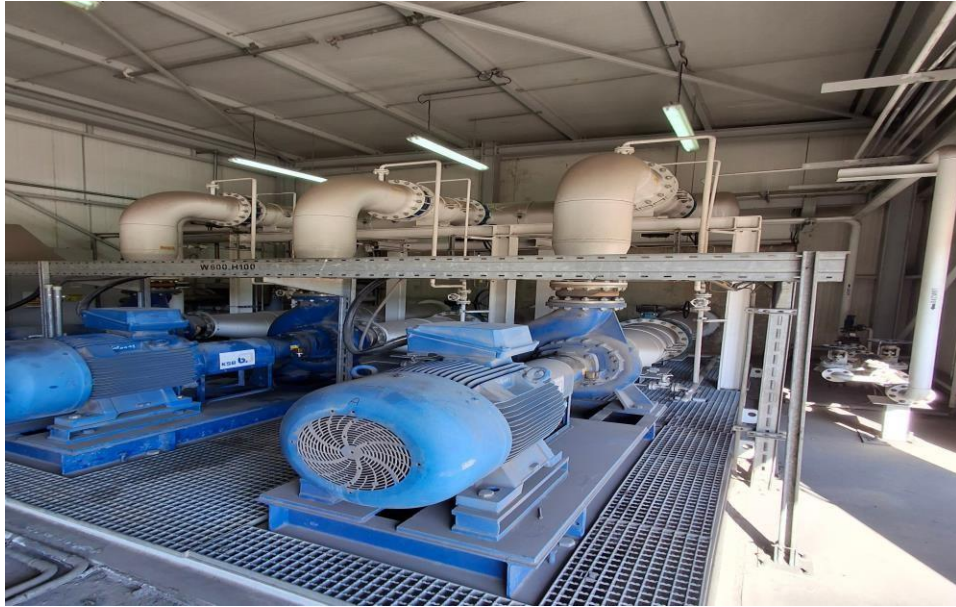
Appendix D.11: Cooling water pumps
