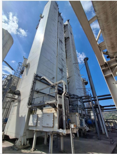
Appendix D.7: Real picture of the distillation column
