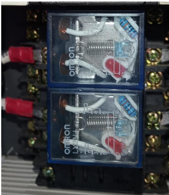
Figure 4. 5: The protection relays
