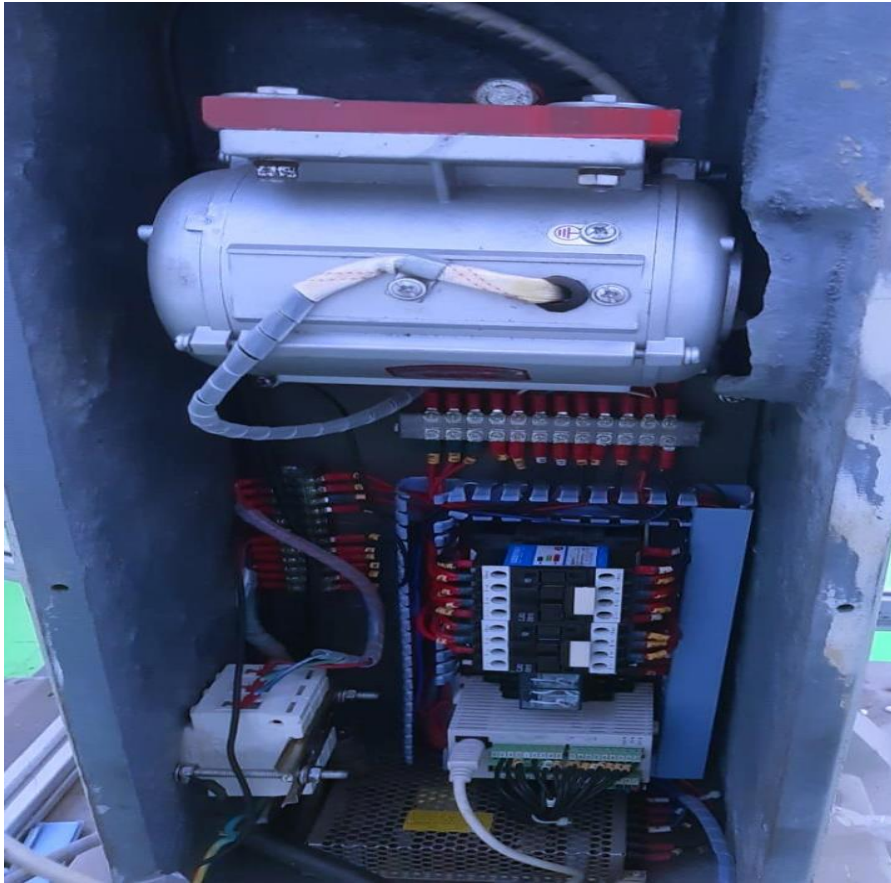
Figure 3. 5: Electrical Control Panel and Motor Assembly within the JBW-300N Impact Testing Machine.
