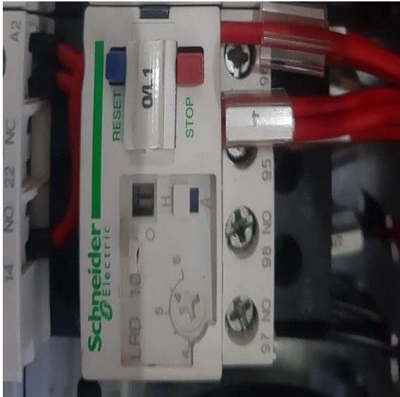
Figure 4. 3: The motor overload relay
