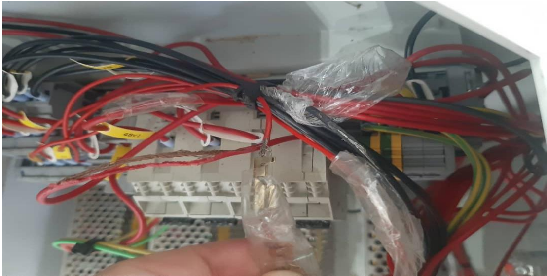
Figure 4. 9: The wiring before correcting its insulation.
