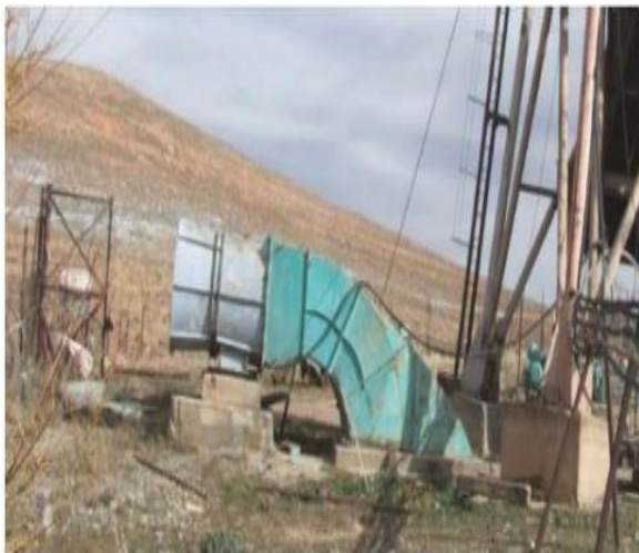
A : Main Exhaust Ventilator [2]
